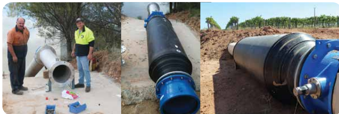
Riverland grape grower Dino Sigismondi, right, starts to install a DELTA SU450 SL501 onto a 450mm pipeline on the Murray River 30 kilometres down river from Loxton, SA. The pipeline irrigates a 121-hectare vineyard.
