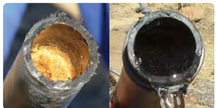
An irrigation pipe blocked with calcium buildup before the water was treated with a DELTA Magnetic Water Conditioner (left) and the same pipe after treatment with a DELTA conditioner.
